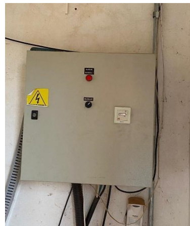
Figura 74 – Painel de controle.
